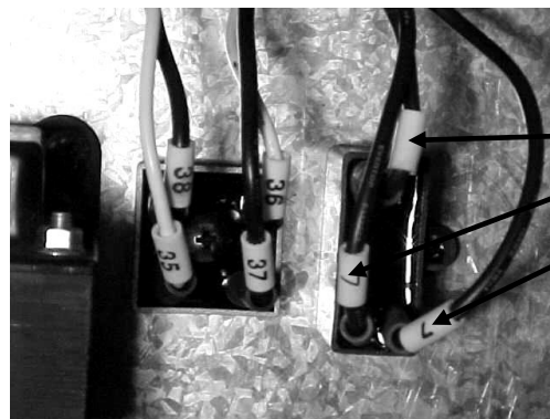
Wires 7, 7 and 43 at C2
